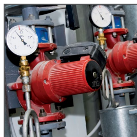
Sensors, valves and control cabinets
