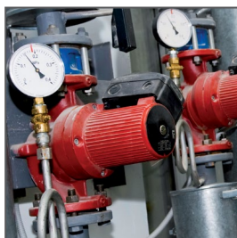
Sensors, valves and control cabinets
