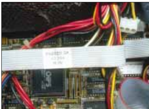
Flat Ribbon Cable Labeling
