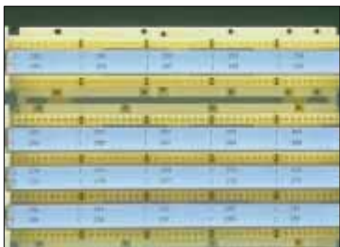
Network Systems Labeling
